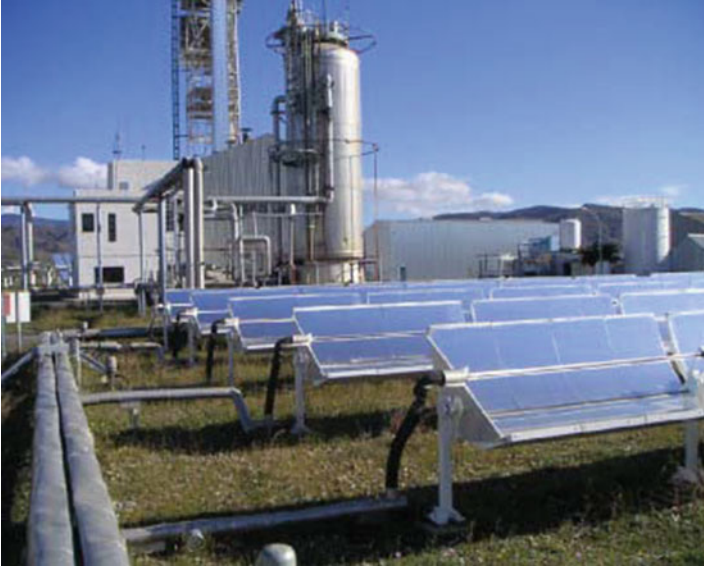
Fig. 2.10 Acurex distributed collector system at the PSA, Spain
