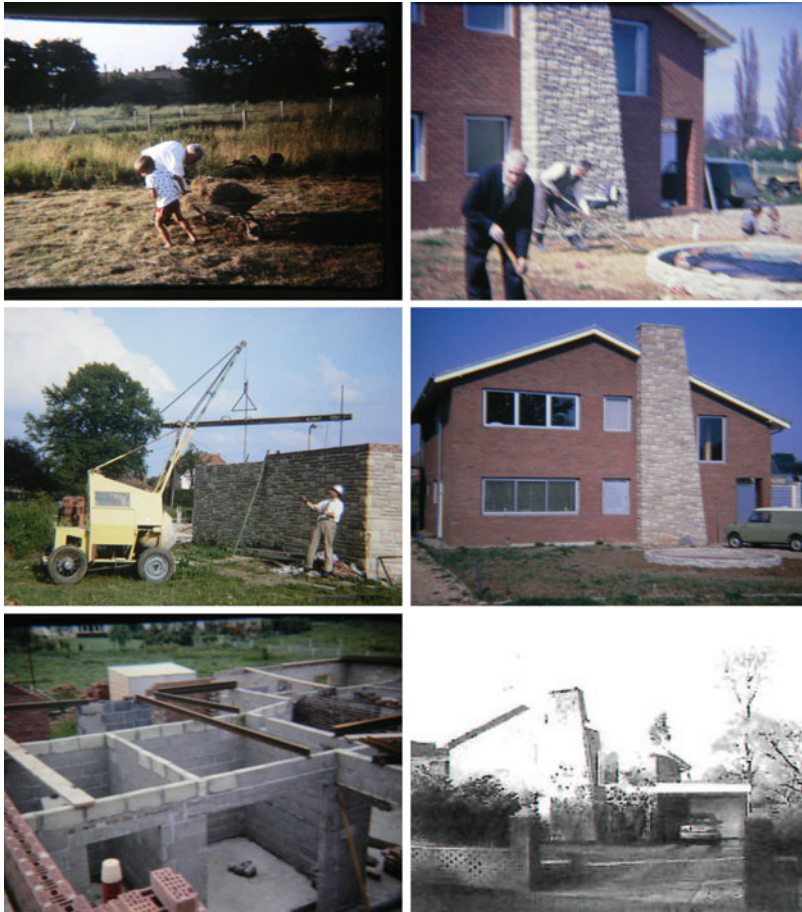
Fig. 20.18 Photographs of stages in the construction of a house by the author, who did all the work except for laying the top waterproof cover on the flat roof over the garage. It took 18 months from start to moving in although not all the rooms were finished. At the time it was the only house in town that had an indoor swimming pool. An essential preliminary test for Mike was the design and construction of a mobile crane and cement mixer. It started life as a Morris 8 car
