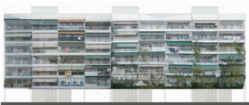
Fig. 8.9 West façade (real photographic reconstruction) of one of the three double building blocks in the Peristeri urban compound
