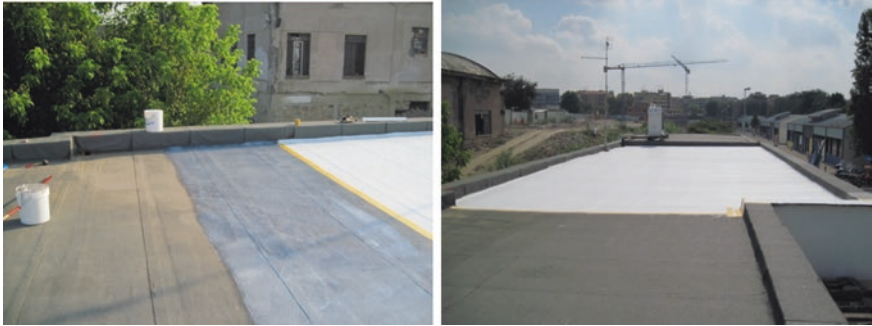
Fig. 20.13 Implementation of a cool roof system in a recreation center in Rome
