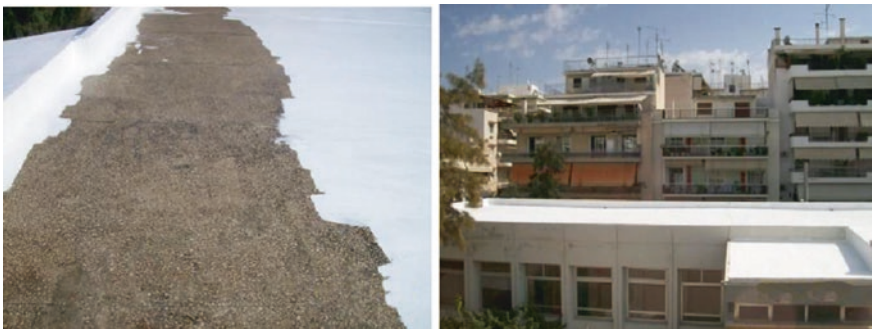
Fig. 20.16 Implementation and completed installation of the cool roof on the Athens school
