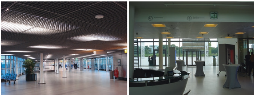
Fig. 22.5 Inefficient lighting solution ( left ), lack of control ( right )
