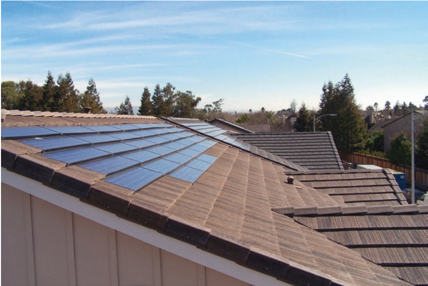
Fig. 18.11 A roof-integrated PV system in San Jose, California (NREL)
