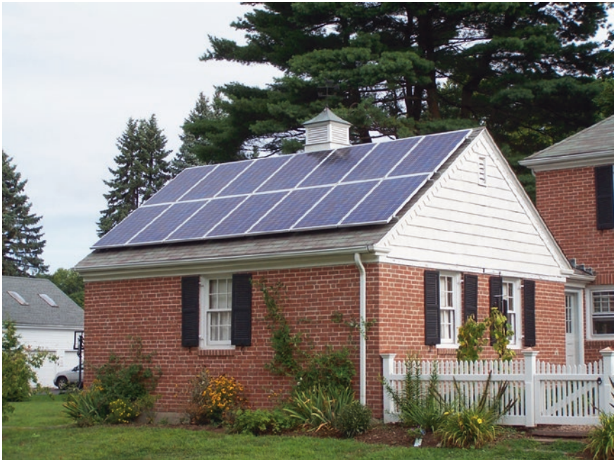
Fig. 18.10 A residential grid-tied PV installation in Glastonbury, Connecticut (NREL)
