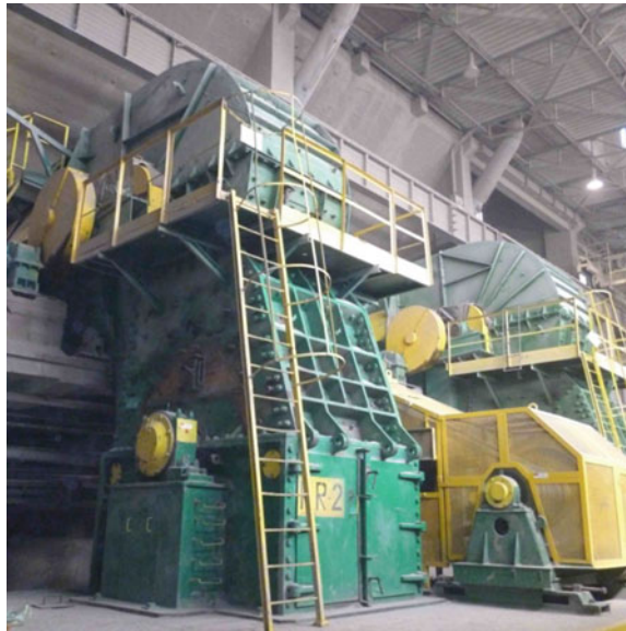
Fig. 1 A crusher—general view (note bearings with yellow housing)
