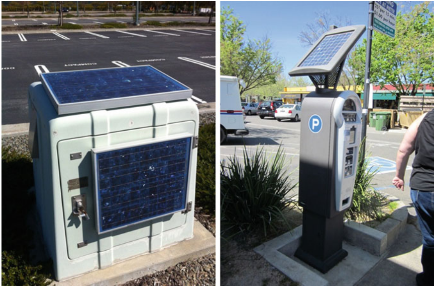
Fig. 9.5 Typical solar power remote monitoring and control devices [25, 26]
