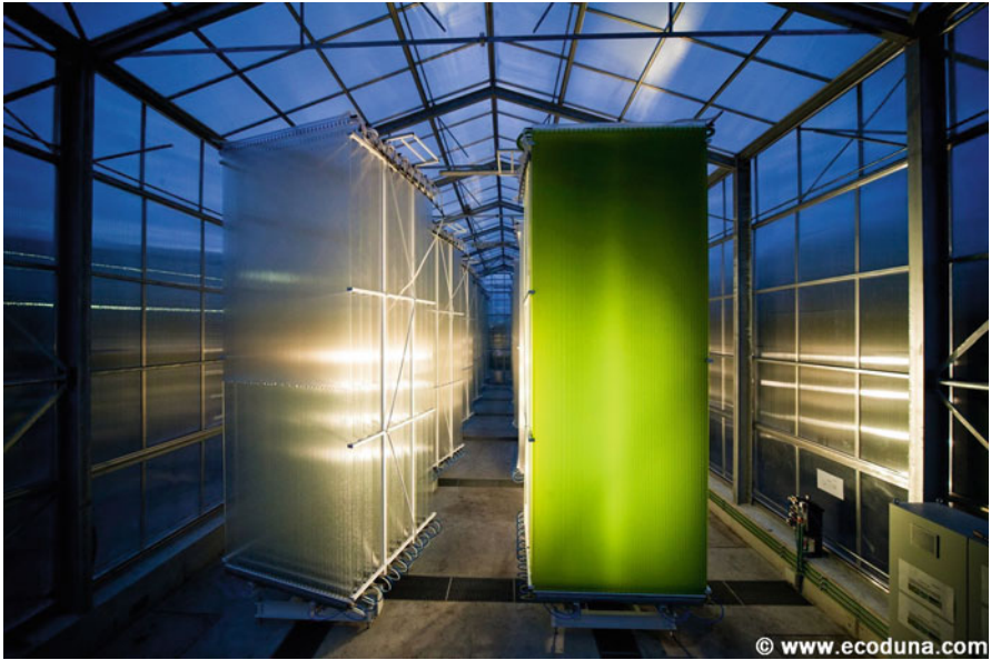
Fig. 15 Indoor operated “Hanging gardens” PBR plant of ECODUNA operated in Vattenfall, Germany (online resource 6; with kind permission of ECODUNA)
