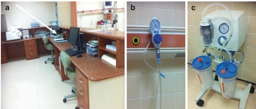
Fig. 6.6 (a) A PACU desk space for physicians and nursing staff to write notes, a telephone line [A white arrow], a computer terminal and a central patients monitor and (b) a bedside and (c) portable suction equipment
