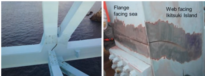
Fig. 2 Photos of the crack found
