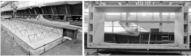
Fig. 13 Deck slab on the casting table left . The finished precast bridge girder right
