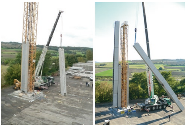
Fig. 5 Auxiliary pier and assembly of compression struts with the aid of a mobile crane left . Assembly of the second bridge girder right
