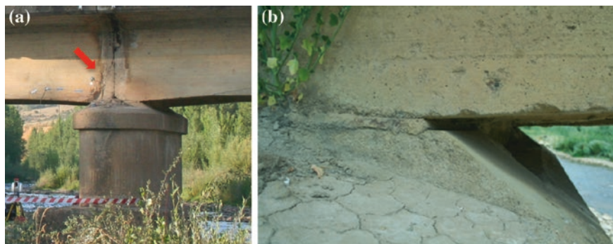
Fig. 4 Supports: a signs of deterioration at the support, b detail of the bearing
