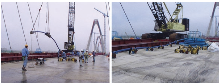
Fig. 14 Stay cable unreeled and lifting up Stay Cable to install on pylon side
