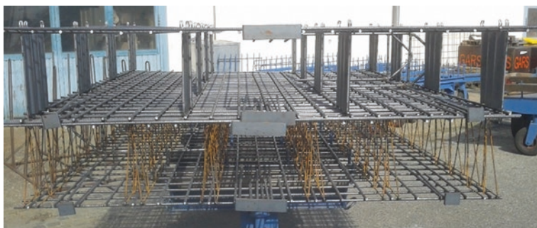
Fig. 11 Reinforcement cages for the hollow wall elements. Top reinforcement cage using curved steel elements. Bottom reinforcement cage using lattice-girders
