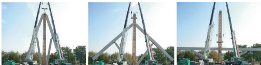
Fig. 6 Lowering of the top points of the bridge girders with the aid of mobile cranes
