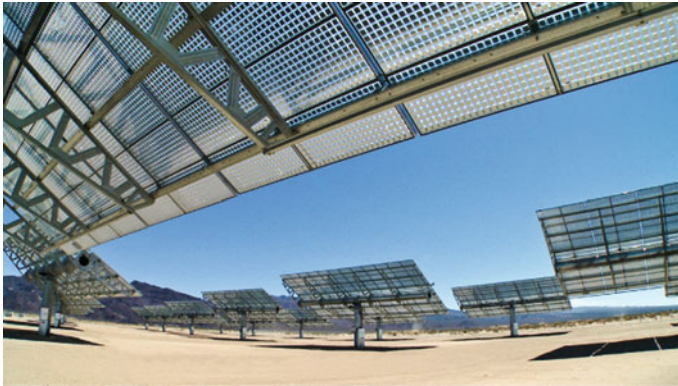
Fig. 3.1 CPV solar farm in Newberry Springs, California, producing 1.5 megawatt. © Soitec
