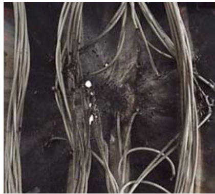
Fig. 6 Image of cable bundles destroyed by an impact
