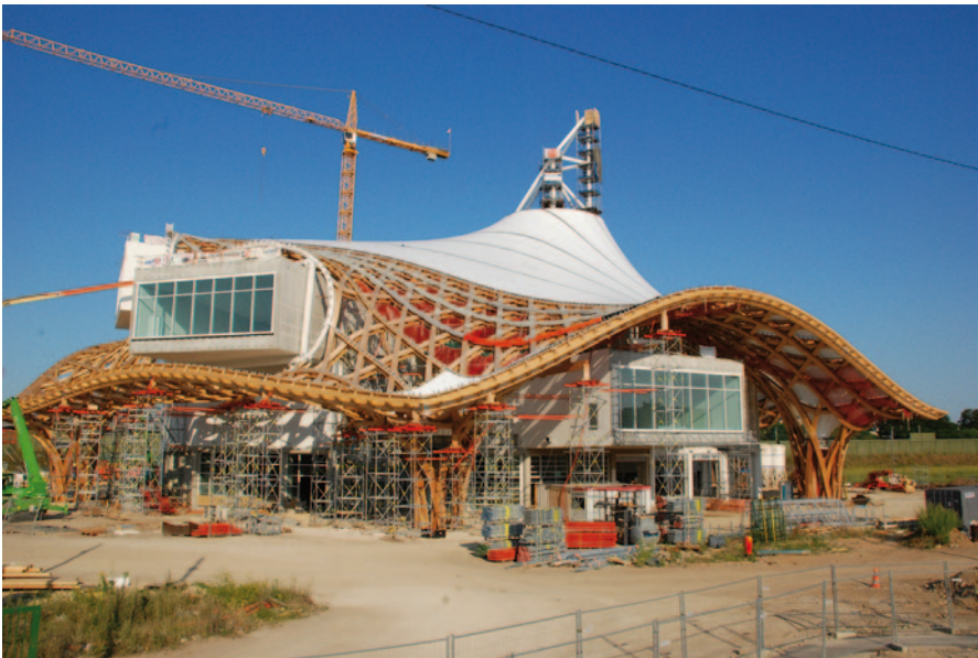
Fig. 3.12 Centre Pompidou in Metz, France, under construction, architect Shigeru Ban. (Courtesy of G. Pohl)
