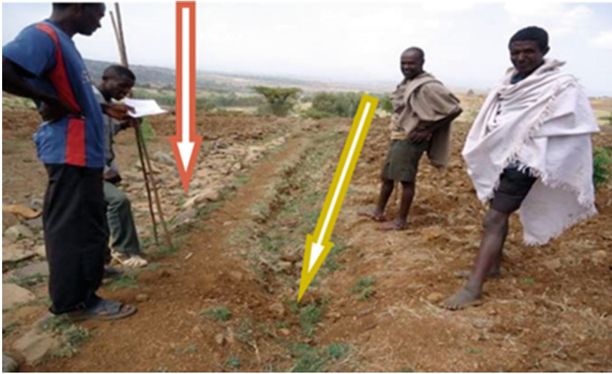
Fig. 35.8 Two waterways constructed side by side along two districts boundary due to land ownership issues and lack of integrated water management
