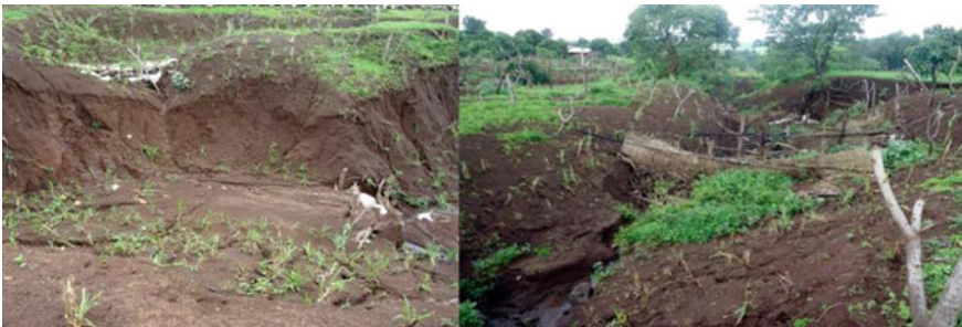
Fig. 35.5 Failed wooden and soil-filled sack check dams
