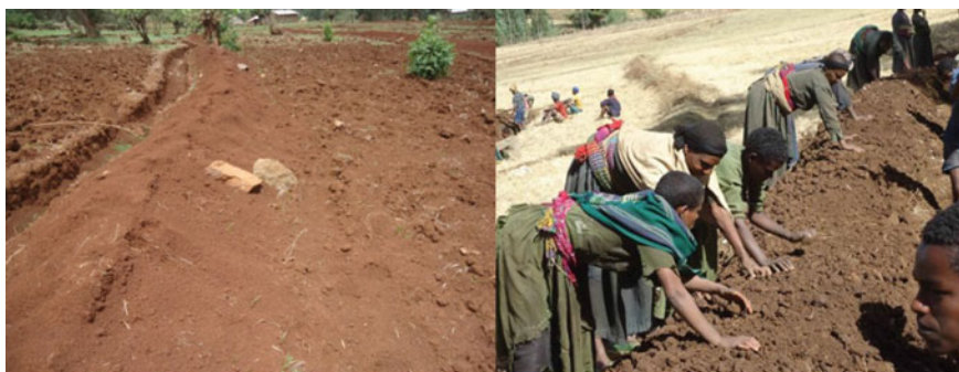
Fig. 35.3 Poorly compacted soil bund ( left ) and bund construction ( right )
