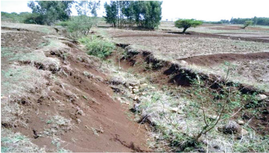
Fig. 35.7 Fragile gully without treatment used as waterway
