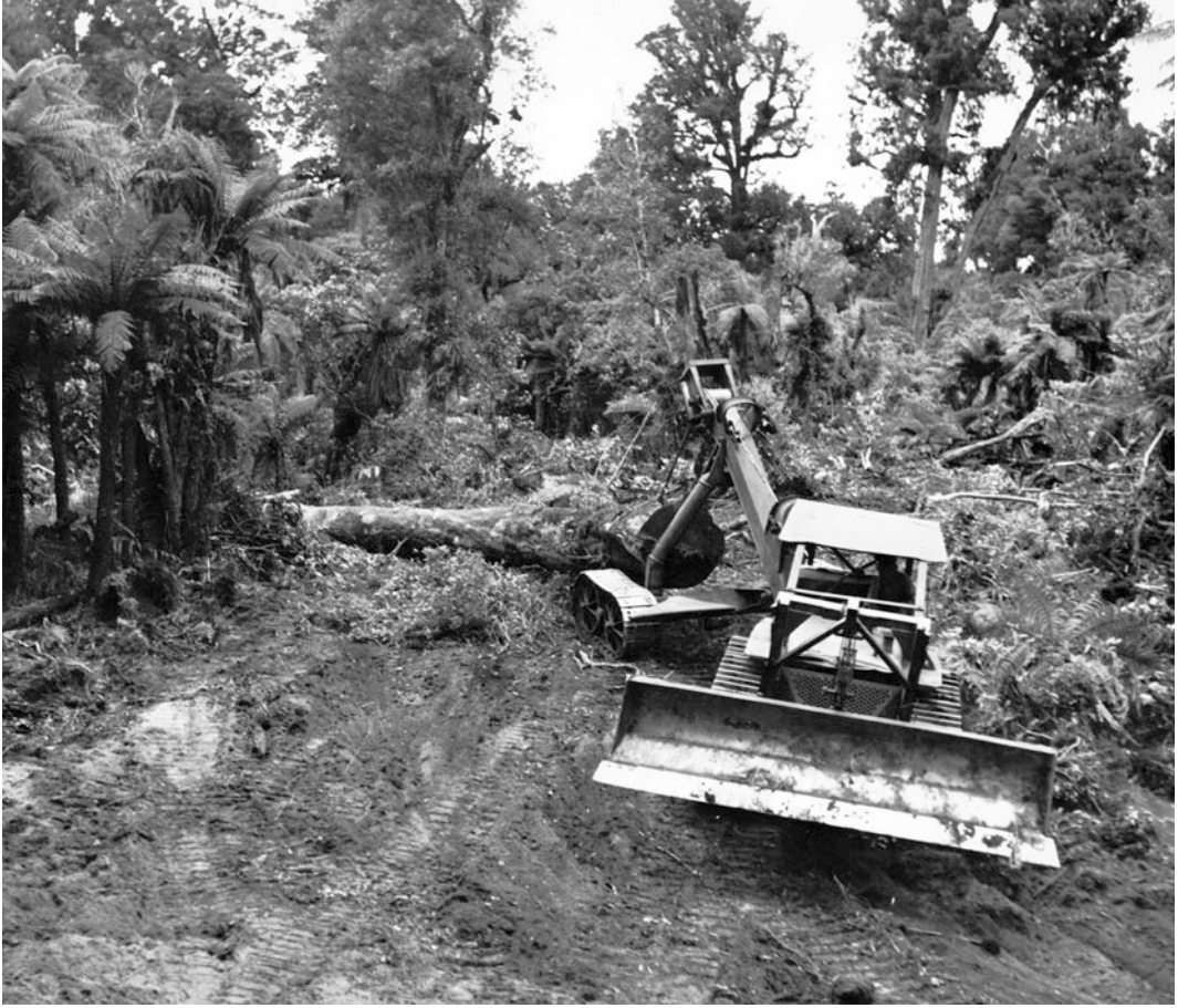
Fig. 7.12 A D8 tractor tows a logging arch, a heavy steel lifting arm on its own caterpillar tracks, at Pureora. The arch lifts the leading end of the log off the ground,
