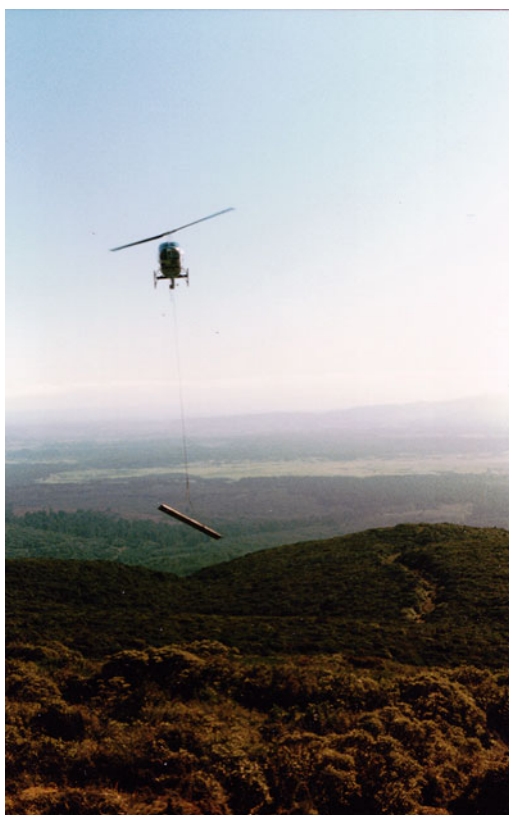
Fig. 14.10 Helicopter pilot Allan Murtagh flies timber up to the summit of Pureora Mountain for repair work on the infamous bulldozer track. Erosion of the fragile pumice soil is a constant problem (See Fig. 1.10). The damage to the lower slopes still shows in the background. Crown Copyright, Department of Conservation Te Papa Atawhai (1984). Photographer: John Mason
