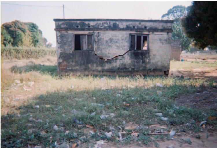
Fig. 16.6 Dilapidated physical structures. This is a deserted house. It is very dangerous, especially for girls because they can be dragged here and violated. These people get hurt ... (Participant 6–16 years old, male, Mozambique)
