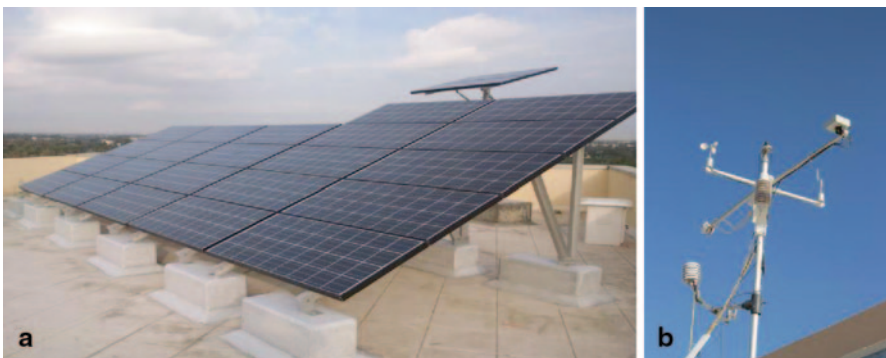
Fig. 48.2 a Installed PV systems; b Installed weather station
