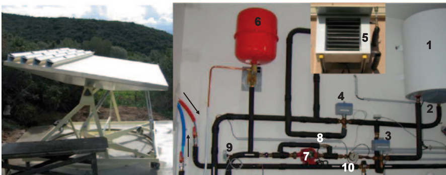
1. Water heater with electrical resistance 2. Temperature sensor (dry cooler gate control). 3. Water heater gate. 4. Dry cooler gate 5. Dry cooler (outdoor). 6. Expansion tank. 7. Pump. 8. Flow rate adjustment. 9. Temperature sensor (water heater gate control). 10. Flow meter
