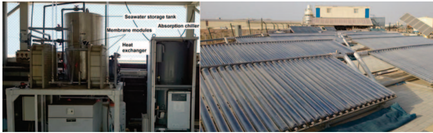
Fig. 71.2 Solar thermal polygeneration unit
