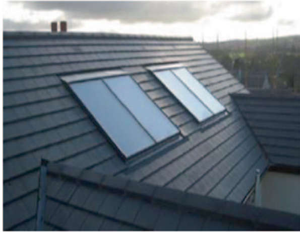
Fig. 64.5 Roof-integrated flat plate building-integrated solar thermal system (BISTS) for solar water heating
