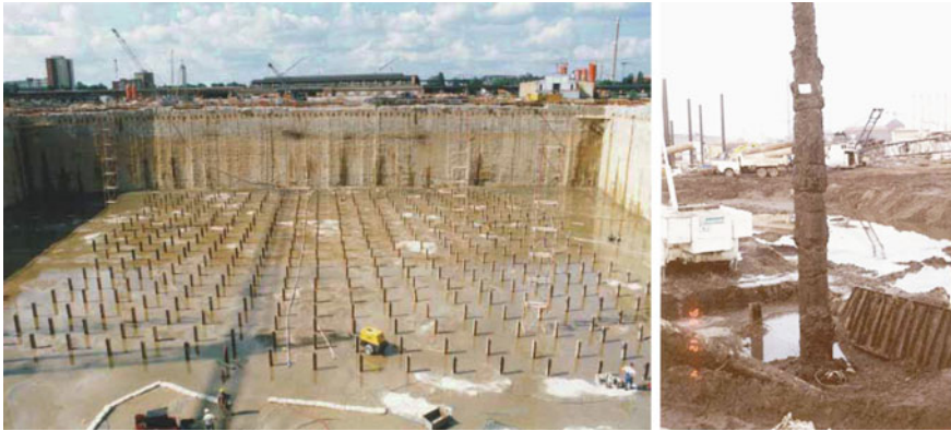
Fig. 1 Grid of vibro-injection piles to tie back an excavation base slab. Deep excavation of about 20 m in urban area ( left ) and recovered pile ( right )
