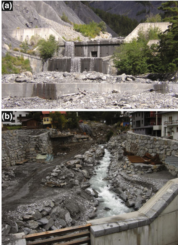
Fig. 12.18 a Grade control check dam in the torrent Le Riou Bourdoux, near Saint Pons in the Ubaye River catchment, French Alps. The works were constructed in the 19th century (photo by S. P. Rice); b Channel construction on a colluvial (debris flow deposit) fan to protect concentrated settlement (Carinthia, Austria). Both views upstream
