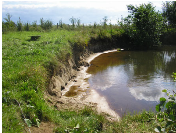
Fig. 14.14 Erosion of outer bank in the Hardebek-Brokelander Au River, in northern Germany (courtesy of Dr. M. Hassan Nasermoaddeli, BAW, Hamburg, Germany)
