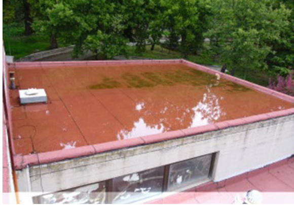
Photo 8 Water-logging on the caretaker's apartment
