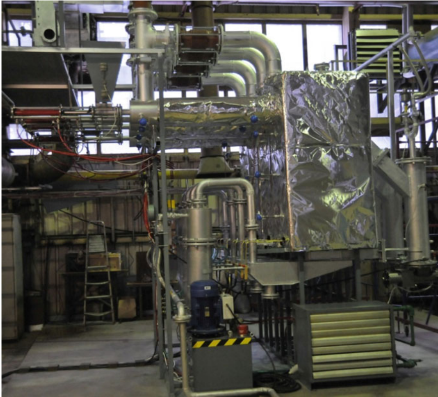
Fig. 3 The power station for production of electrical energy from biomass with capacity 50 kW
