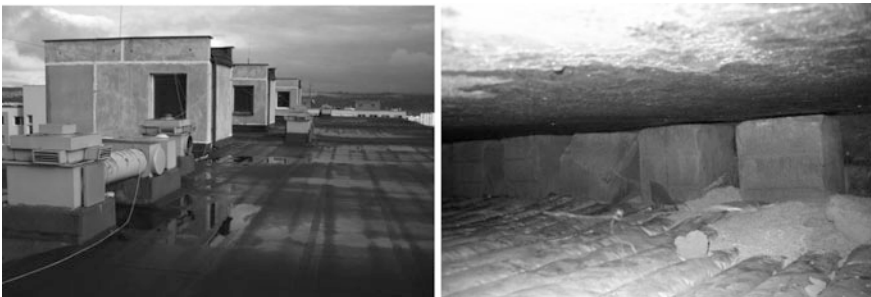
Fig. 2 Views above and below the air gap of the P 1.14/15 construction apartment block
