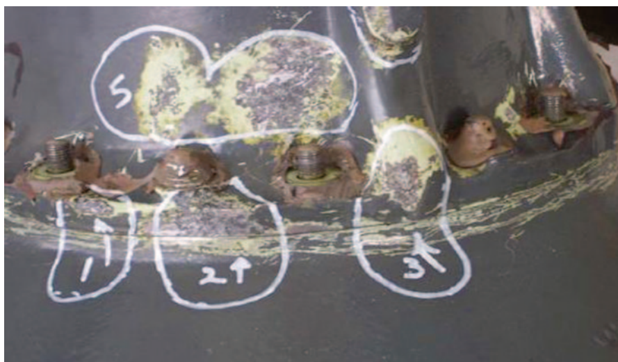
Fig. 10.3 Corrosion locations on a H-53 tail gearbox housing. (Leyman and Champagne 2008)
