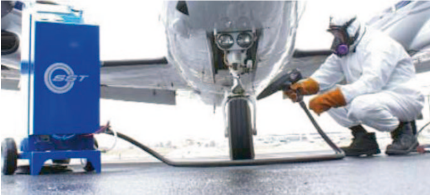
Fig. 10.22 On-site cold spray aluminum repair of IVD aluminum coating using a portable cold spray system. (Birtch et al. 2008)
