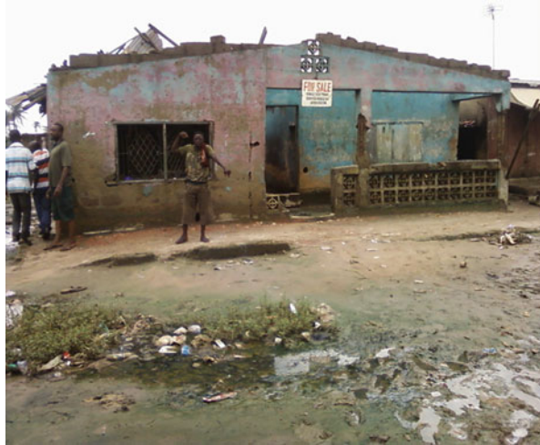
Fig. 7 A dilapidated house at Ikosi (Source: authors, June 8, 2011)
