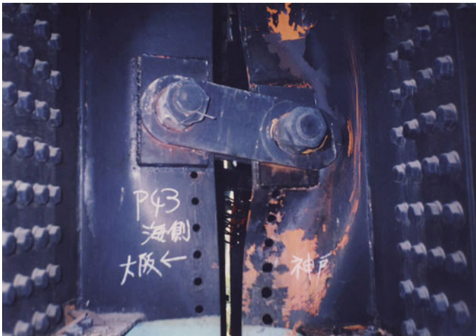
Fig. 1.3 Local damage at the ends of superstructure segments (Kobe earthquake 1995)
