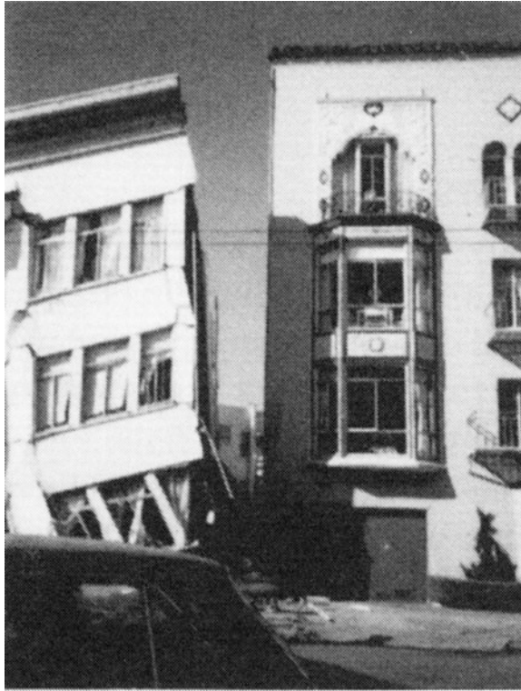
Fig. 1.2 Collapse of a building (Loma Prieta earthquake, 1989) (reprinted from Kasai and Maison 1997 with permission from Elsevier)
