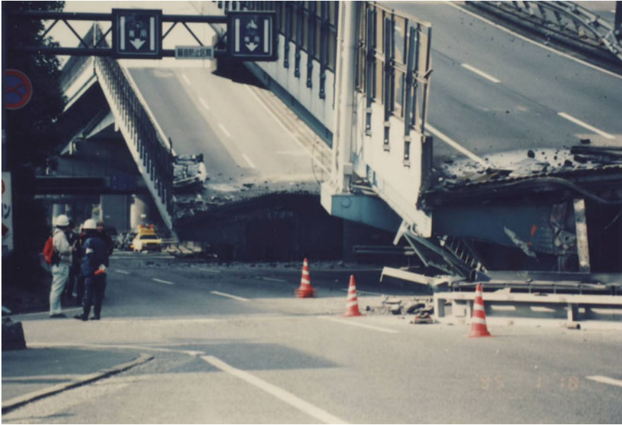
Fig. 1.4 Pounding as one of the reasons for falling down of superstructure segments (Kobe earthquake, 1995)
