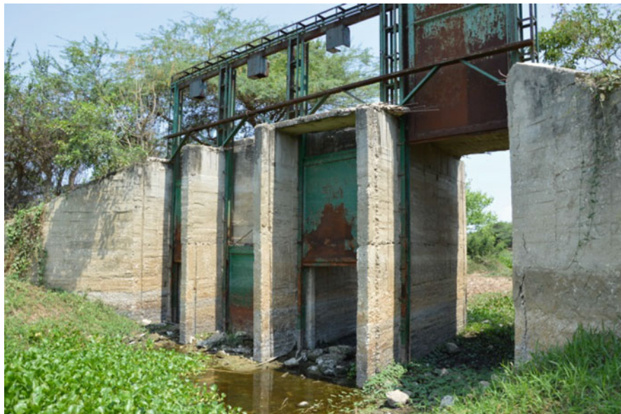
Fig. 8.3 Example of gates for flood control. Photo: Fabio Amador
