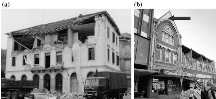
Fig. 7 Examples of out-of-plane collapse mechanism: a wall of the top floor [22]; b parapet and wall collapse and successful strengthening with ties ( arrow ) [23]
