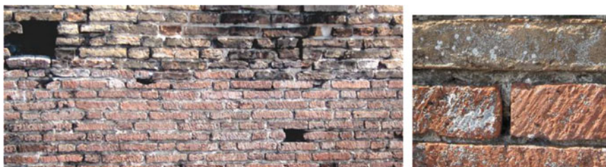
Fig. 6 Change of the surface workmanship at about 8.0 m from the top of the tower (the bricks of the lower portion are superficially scratched)
