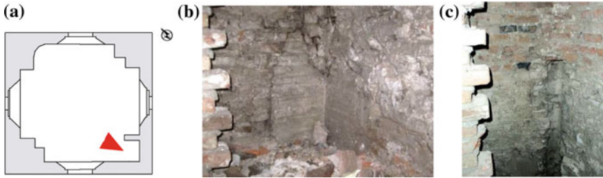
Fig. 10 Details of the South corner at level 4 (a): b the corner is partially dismantled with a probable infilled merlon and c with an embedded pipe at the edge
