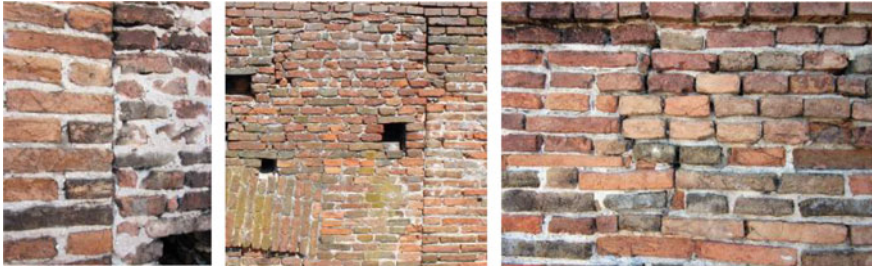
Fig. 8 Typical discontinuities on top of the tower and lack of horizontality of the masonry courses
