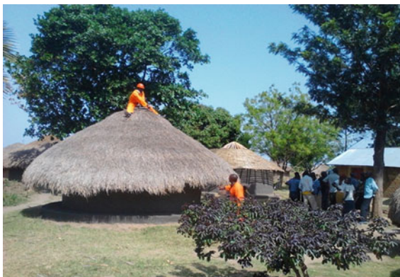
Fig. 15.1 Installation of LUAV micro-solar systems in a village by Barefoot Power Uganda
