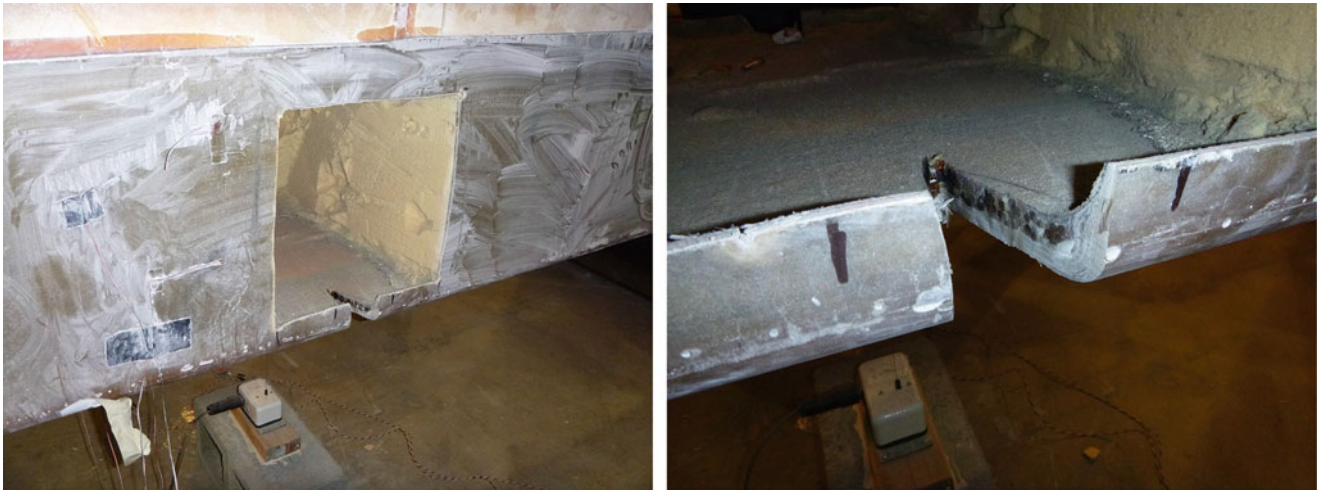
Fig. 22.3 Photographs of damage introduced to beam through cutting of prestressing strands (symmetric cuts on both sides of beam)
