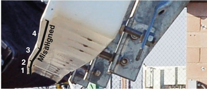
Fig. 12 Bottom-right view of misaligned HCPV modules
