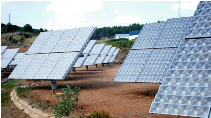
Fig. 23 Magpower HCPV power plant (courtesy of MagPower)
