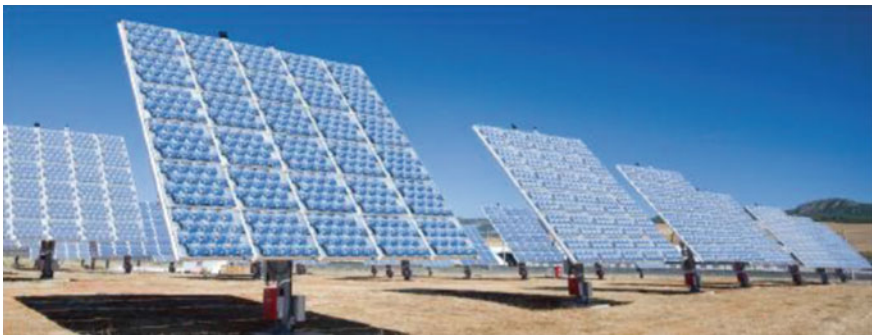
Fig. 22 Solfocus/ISFOC HCPV power plant ( courtesy of Solfocus/ISFOC)
