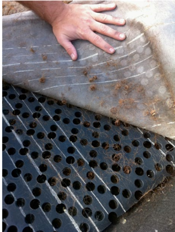
Fig. 3.1 Four-year old roots on a destructed green roof passing through root barriers into drainage/retention layer. (Mark Simmons)
