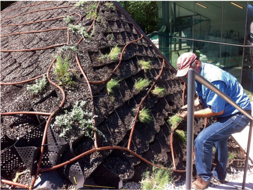
Fig. 16.19 Custom soil with cabled slope revetment geotextile, drip tube, and plant installation on the roof during construction. (Mark Simmons, Ecosystem Design Group)
