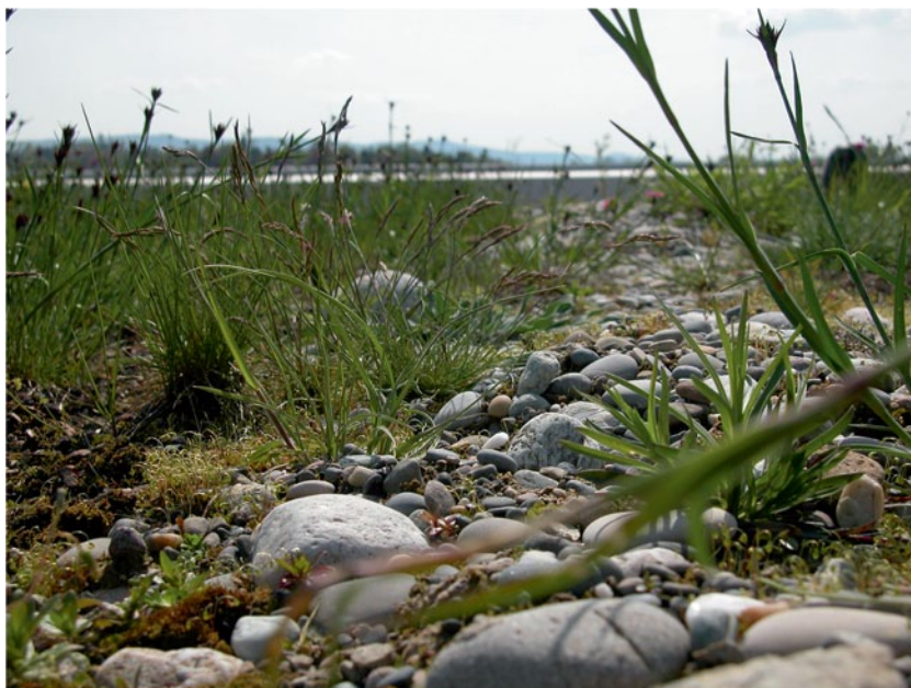
Fig. 16.16 Dr. Stephan Brenneisen determined that various size stones, gravel, bare spots and a variety of vegetation forms are ideal habitat characteristics on green roofs for attracting wildlife. Monocultures and even substrate depths on green roofs can be beneficial to some wildlife, but the diversity in materials, structure and arrangement offers variety, cover and choice. (Stephan Brenneisen)
