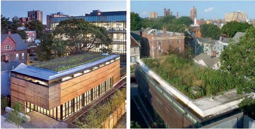
Fig. 12.1 The green roof at Yale School of Art Sculpture Gallery was left undisturbed for 6 years after establishment. Vegetation at time of planting ( left ) and after 6 years of growth ( right ). (Left Image by Peter Aaron, Right Image by KieranTimberlake)
