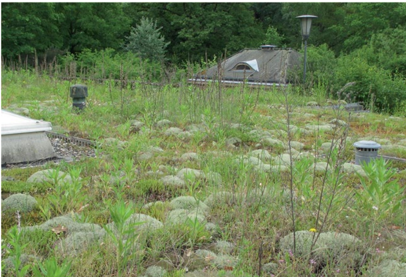
Fig. 16.22 The 130-year-old ruderal green roof in Berlin, Germany has been colonized over the years by moss, lichen, grasses and over 50 species of herbs. After the green roof was removed, stockpiled, and restored in 2005, the same plant communities re-colonized the roof. (Kelly Ksiazek)
