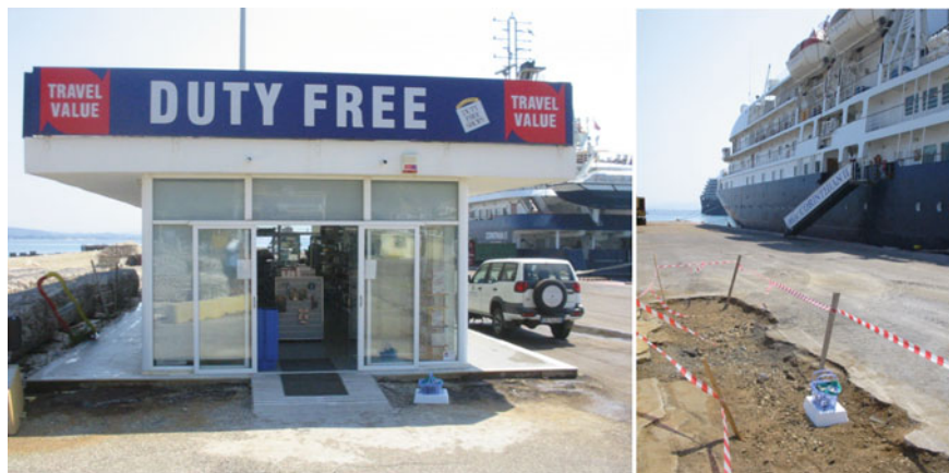
Fig. 6.1 The damage of asphalt cover due to the seepage of CH 4 and H 2 S rich gas at the tourist harbour of Katakolo (western Greece). At the step of the Duty Free Shop's door the H 2 S concentration in air a few cm above the ground can reach hundreds of ppmv. The white box on the ground is an accumulation chamber for measurements of gas flux. The site on the right photo is approximately located where an explosion occurred in 1972 (photos by G. Etiopie)
