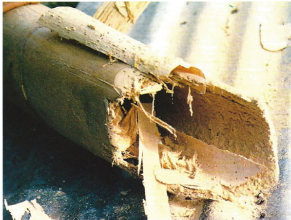
Fig. 9.10 Culm deterioration by termites (Liese and Kumar 2003)
