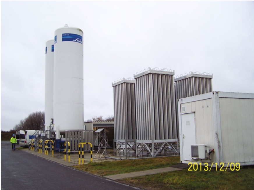
Fig. 4 Injection facility at Ketzin with two intermediate CO 2 storage tanks ( left ) and ambient air heaters ( middle ) before decommissioning in December 2013
