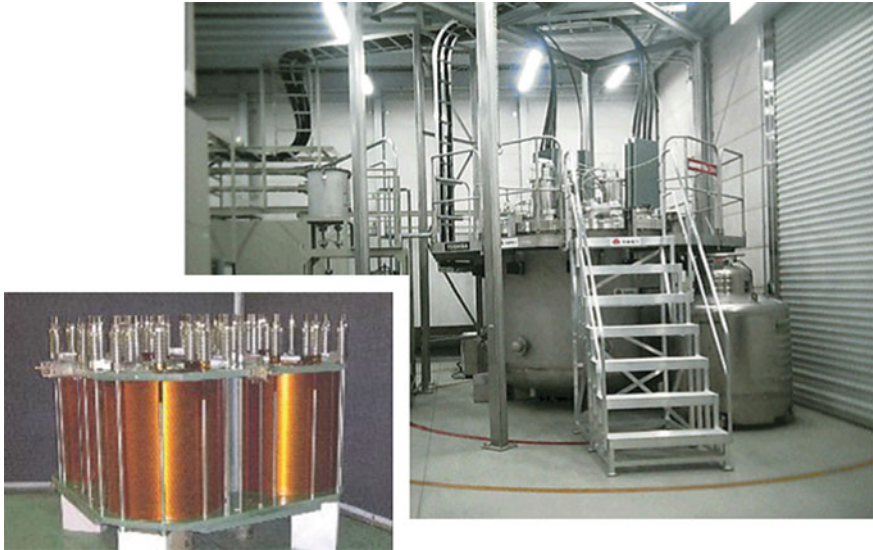
Fig. 10.15 A 5 MVA SMES system with four pole solenoid design, built by Chubu Electric Power and Toshiba Corp. Power System Co. Japan. The inset on the left are the four pole superconducting magnet Coils [36] (With permission from Elsevier)
