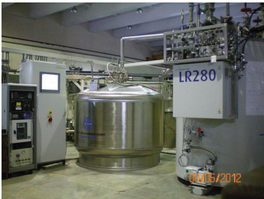
Fig. 1.8 A modern day turbine based helium liquefier with a refrigeration capacity of 900 W ( \sim 300 l/h) manufactured by Linde Kryotechnik AG installed at IUAC in 2012 (Photo courtesy IUAC Delhi)
