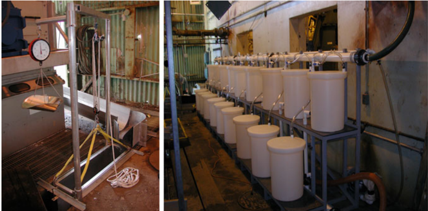
Fig. 4.2 Impingement sampling equipment used inside a screen house ( left )—traveling water screen housing is at left with fish return trough exiting through the side; collection basket is suspended in discharge of return trough. Post-collection latent impingement mortality holding system ( right )
