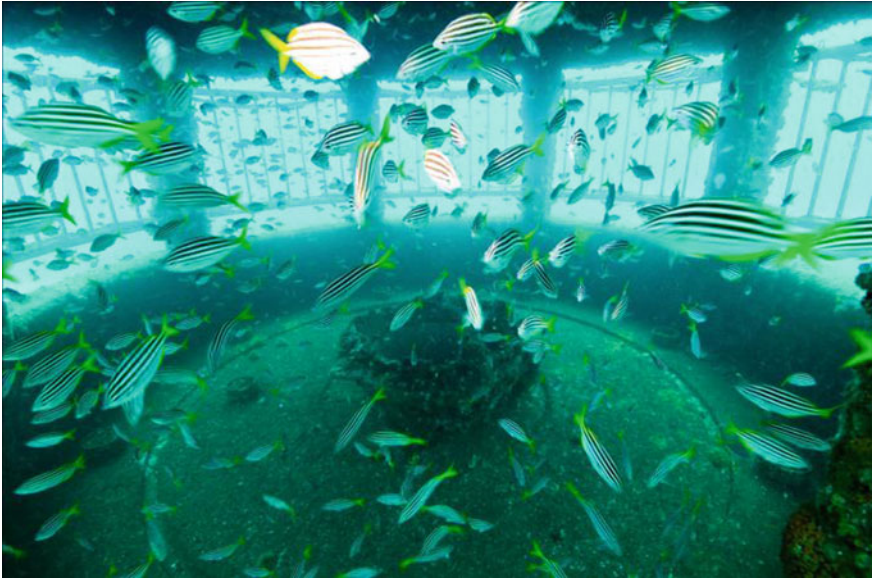
Fig. 3.9 Interior view of the velocity cap intake during operation of the Sydney SWRO plant
