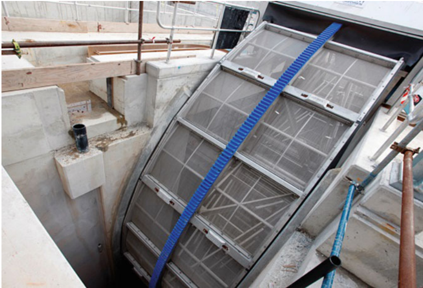
Fig. 3.7 Sydney SWRO plant intake drum screens
