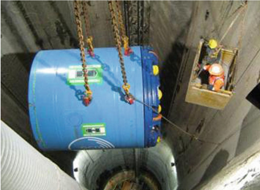
Fig. 3.12 Lowering of tunnel boring machine into the riser shaft connecting the SWRO plant to the tunnel
