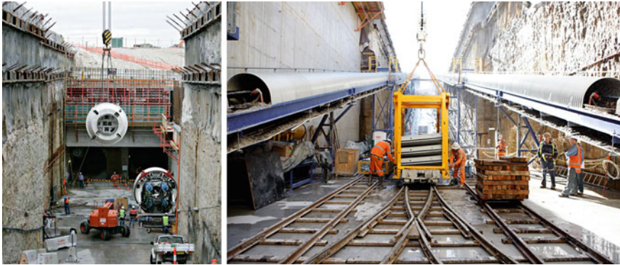
Fig. 2.11 TBM assembly within the “box-cut” leading to the tunnel portals/hauling railway and spoil conveyors leading out of the “box-cut”
