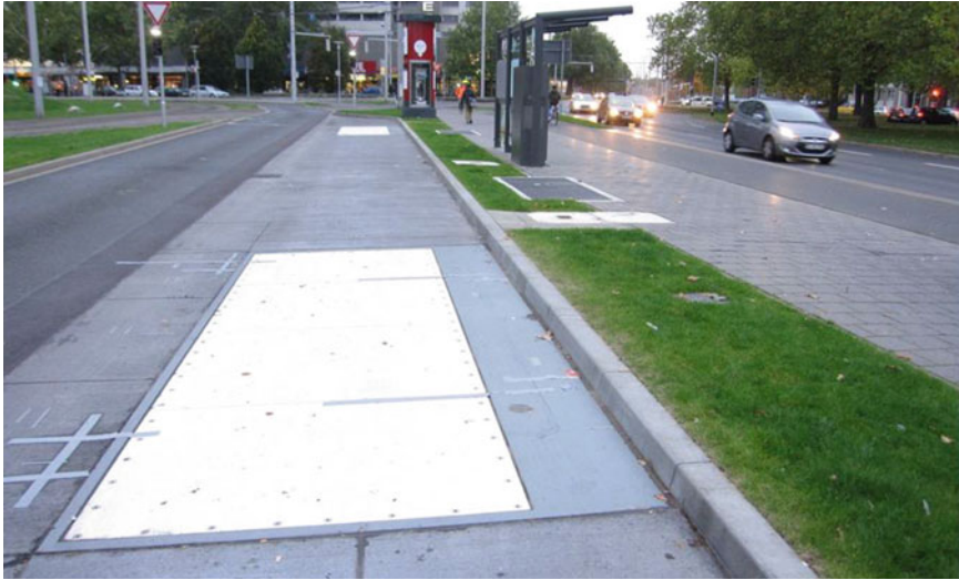
Fig. 2 Inductive charging system for buses at main train station, Brunswick, Germany (Photos by IAV)
