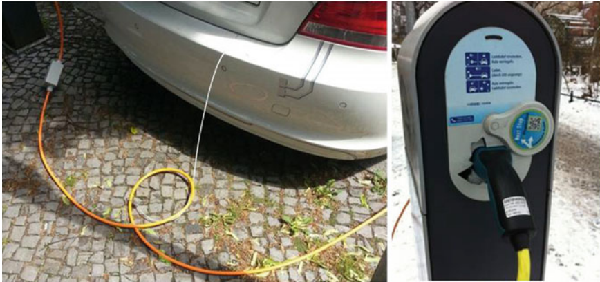
Fig. 7 Cable lock in electric carsharing and damaged charging station (Photos by IAV)
