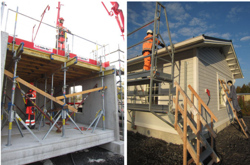
Fig. 3 Specific details at training points. Good practices related to floor casting and floor supports (Training point 2, left ) and proper scaffolding (Training point 30, right )
