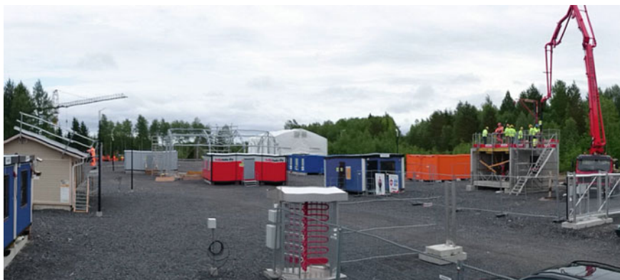
Fig. 1 An overview of the Training Park in Oulu. In this picture (in the left side ), a group of workers is being trained at the construction work for foundations and framework training point
