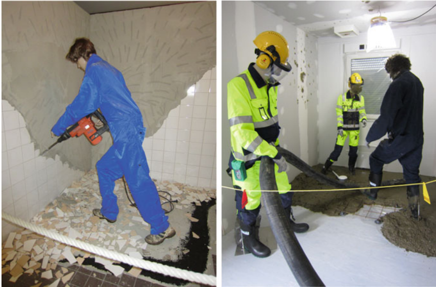
Fig. 2 Training points. Incorrect working methods and inadequate personal protection for chipping old lavatory wall (Training point 8, left ) and the casting of a floor (Training point 6, right ). The dark clothed manikins represent incorrect working methods and inadequate personal protection, whereas the other two manikins represent correct working methods and equipment
