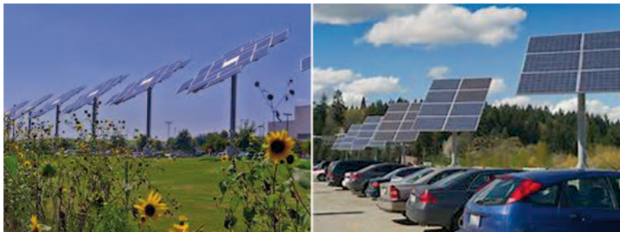
Fig. 12.18 Ground-mounted solar photo-voltaic panels. (© University of Washington Bothell, 2013)
