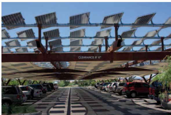
Fig. 12.19 Solar PV shades parking lot in Las Vegas. (©Solar Done Right, 2013). PV photovoltaic
