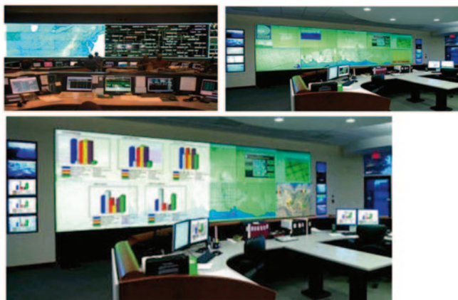
Fig. 12.37 Central Communications Command and Control Center. (© Paul Bierman-Lytle 2009)
