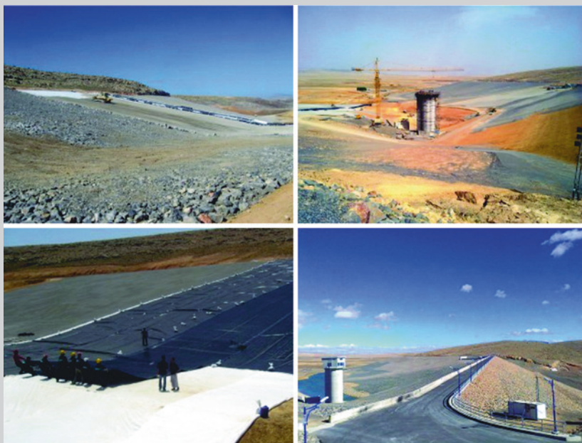
Fig. 16.12 Photos from the phase of impermeable carpet installation (geomembrane and geotextile) http://www.hidrotehnika.rs/alzir/brana-ourkiss/
