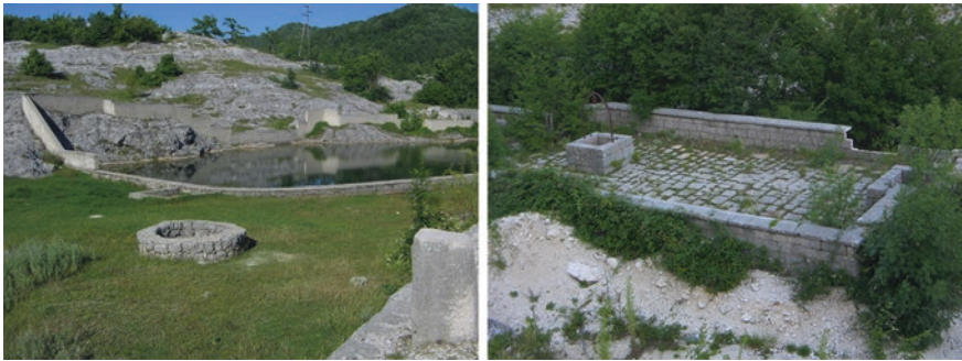
Fig. 2.4 Cisterns—specific reservoirs and intake wells for collecting rain water in high karstic mountains of Montenegro (Vilusi site left , and Grahovo village right )
