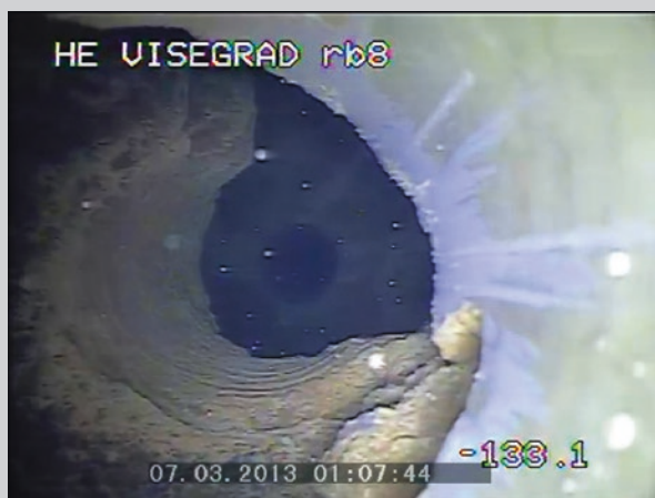
Fig. 16.16 Entrance to cavern at the depth of 133 m from an altitude 337 m a.s.l (video endoscopy)
