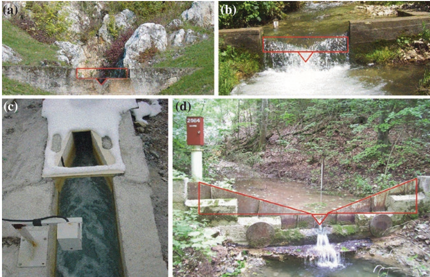
Fig. 7.4 Various types of weirs used for discharge gauging of karstic springs a combined Thomson ( V-notch ) and Poncelet ( rectangular ) weir—dry period; b combined Thomson ( V-notch ) and Poncelet ( rectangular ) weir—wet period; c Parshall flume; and d combined V-notch weir
