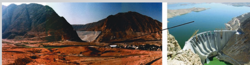
Fig. 16.2 Photo of dam site during construction and Salman Farsi Dam in the last stage of building
