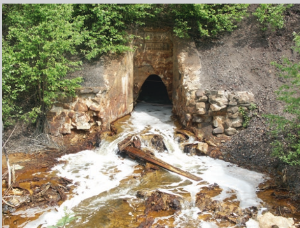
Fig. 16.29 Gravitational discharge of acidic mine water from the Kalinin Mine
