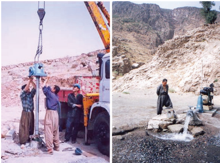
Fig. 11.20 Installation ( left ) and operation of turbine vertical pump in well tapping Qamchuga limestone Fm. in northern Iraq
