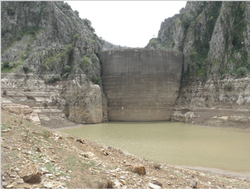
Fig. 13.8 Montejaque Dam, Spain. Abandoned dam due to huge leakage through the heavily karstified dam site and reservoir banks. Photo P. Milanović
