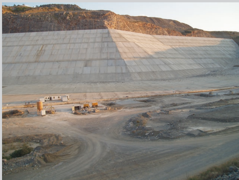
Fig. 13.7 Akkopru reservoir, Turkey. Construction of heavy reinforced concrete slab to prevent leakage through the number of large vertical karst shafts. Photos P. Milanović
