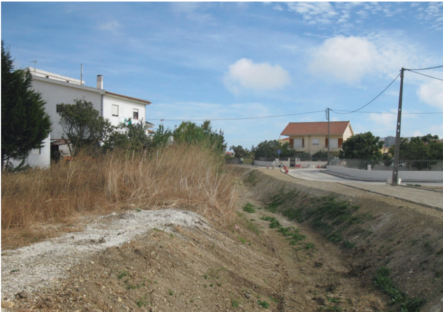
Fig. 7 The measures implemented 2013 for flood protection in the Sassoeiros stream. Without any other measures, e.g., settling adequate plants, the water flow will wash the banks away in the next rain. Photograph Smaniotto (2013)
