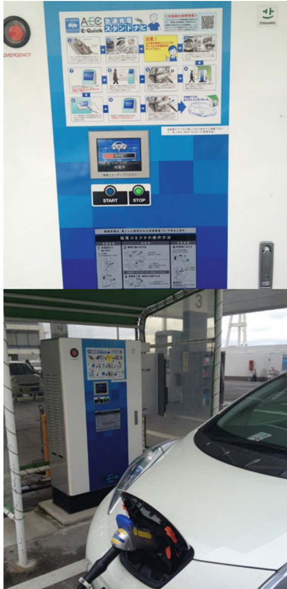
Fig. 2 AEC fast-charging stations (close-up, right ; with Nissan Leaf, left )
