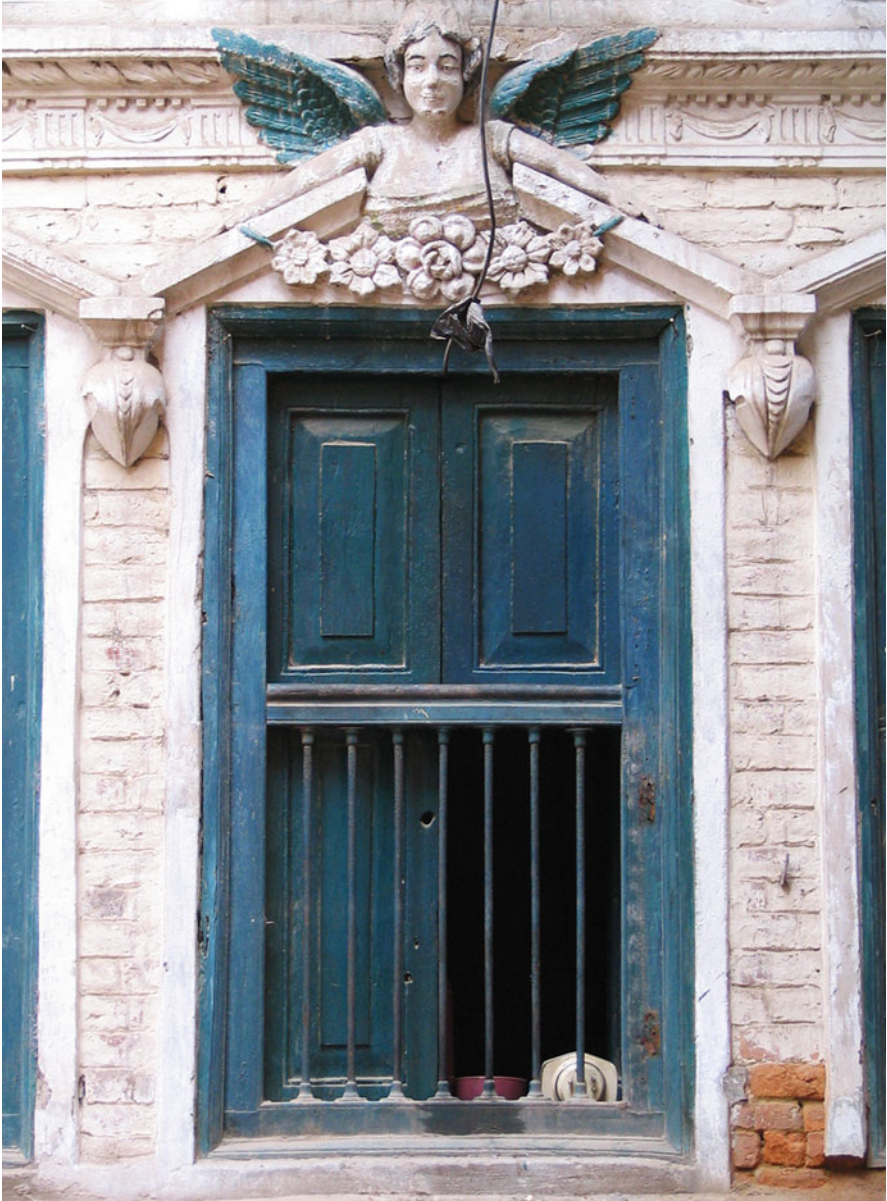
Fig. 8 Patan, Mahāpal (after 1934). A female angel holding a flower garland is cleverly incorporated into the triangular pediment above the central window on the first floor of a residential building. Her wings resemble those of birds. Photo by Katharina Weiler, November 2006
