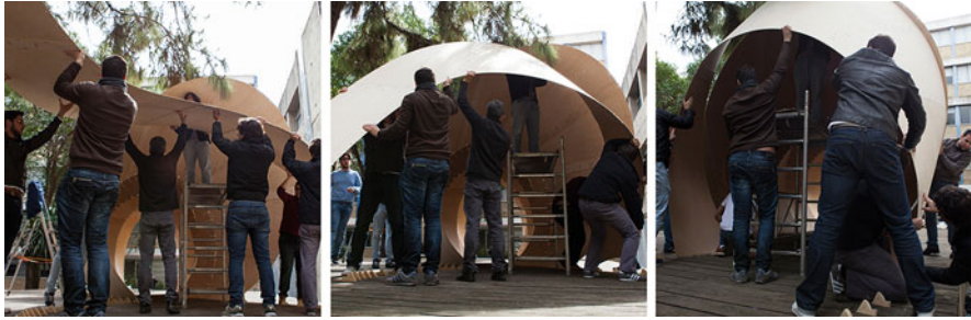
Fig. 13 Left : transportation of the unfolded surface to the installation place. Middle : bending of the surfaces. Right : final bending of the surface and installation of ties
