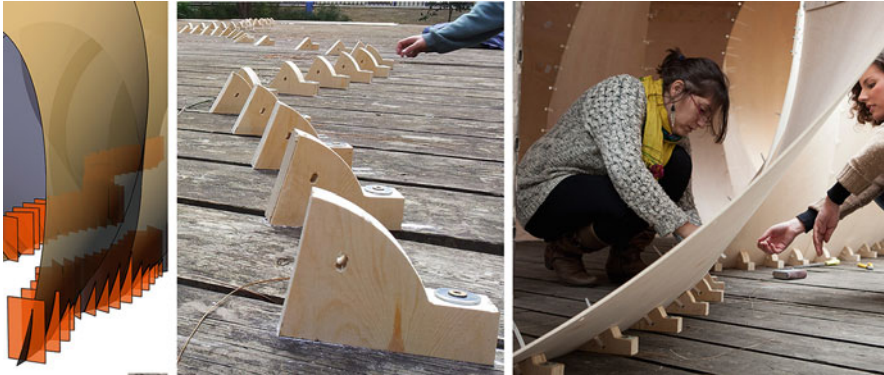
Fig. 11 Left : auxiliary sectioning planes (in vertical position) to determine the shapes of the wedges. Middle : photograph of the definite position of the wedges after setting out with the total station and the full-scale templates. Right : installation of nylon cable ties to link the wooden surfaces to the wedges
