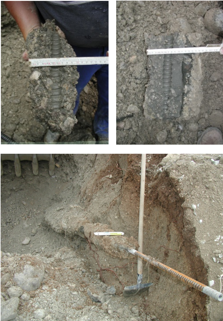
Fig. 1. The diameter of the grout is not uniquely defined and can change consistently along the nail axis
