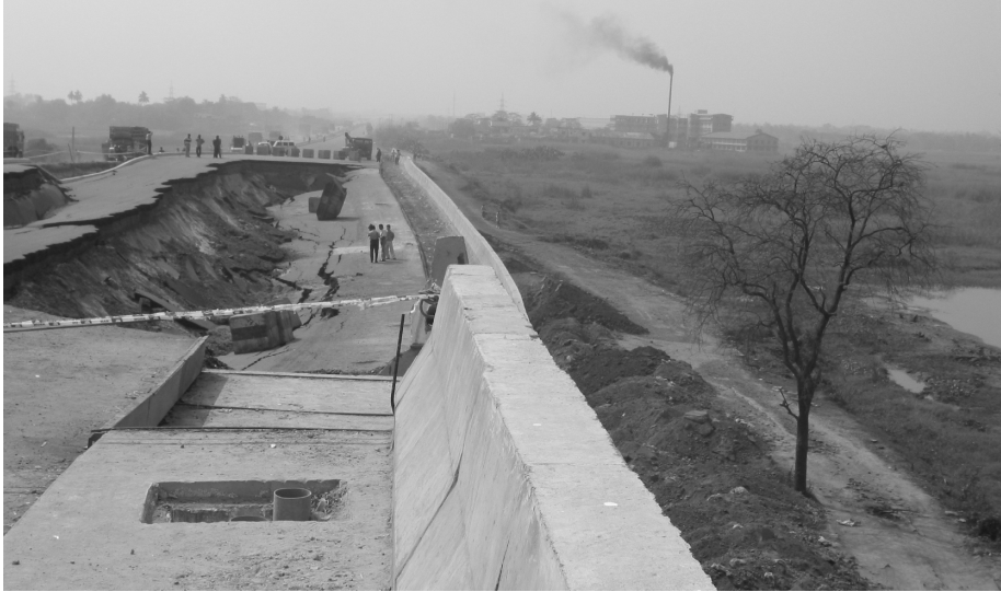
Fig. 1. Embankment Failure adjacent to a bridge approach at Dankuni, West Bengal (India)
