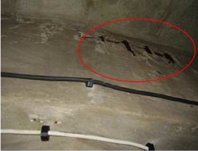
Fig. 2. A crack in the water storage tank's wall
