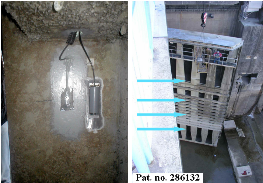
Fig. 4. Strain sensor installation on steel gates of Gabčíkovo Water Power Plant (Slovakia). Left: underwater location of the magnetoleastic sensor with plastic mechanical cover. Right: four sensor installation points on the gate (indicated by arrows) spaced vertically 10 m apart.
