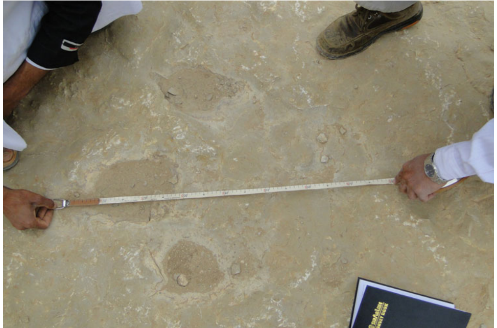
Fig. 19 Decay of limestone rock as a result of the interaction between water and limestone beds
